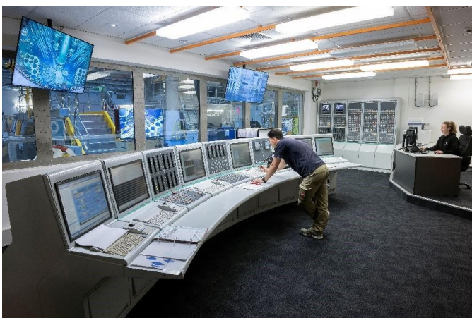
Left: Inside the OPAL control room
