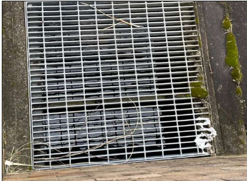
Figure 2.2: Ponding/ Trapped water in pit
