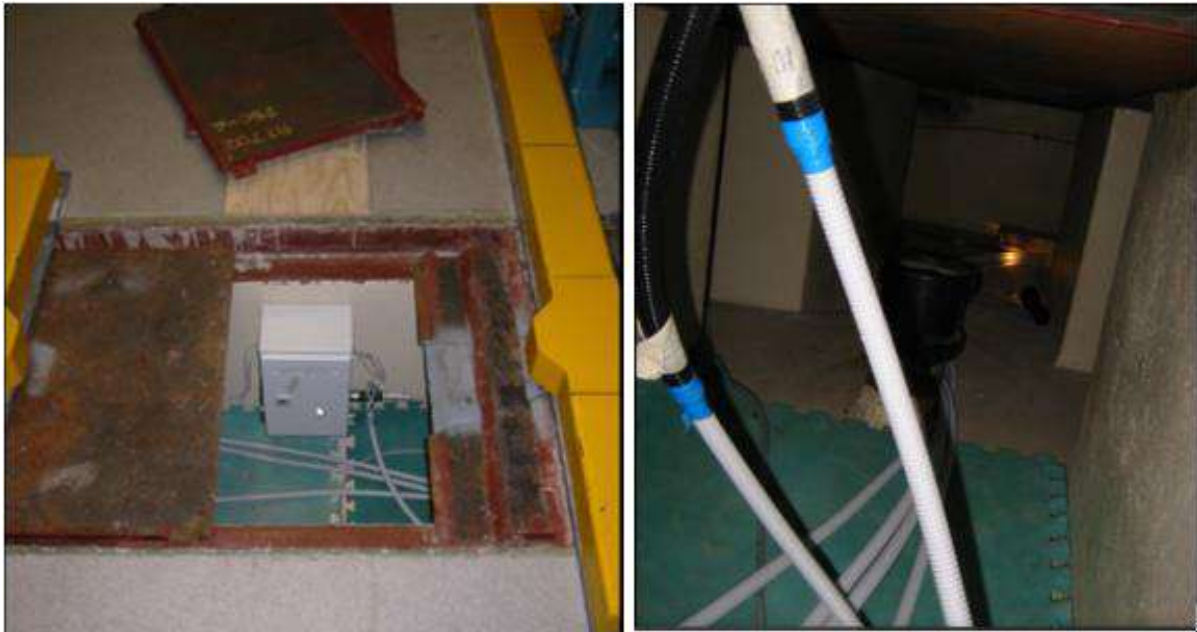
Figure 4 Transfer lines underneath GMP hot cells
