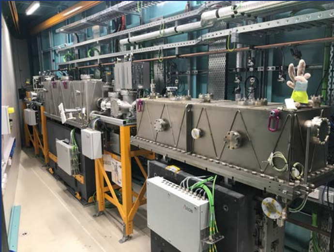
MCT - Hot commissioning of the Photon Delivery System
