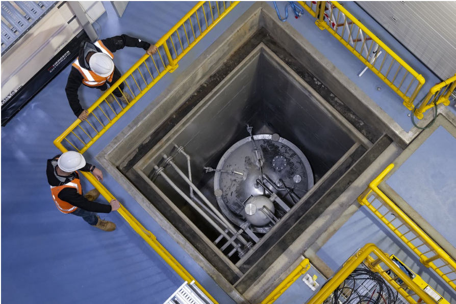
Waste transfer bunker which houses the liquid waste tank in the new ANSTO Synroc® treatment plant, currently in pre-commissioning.
