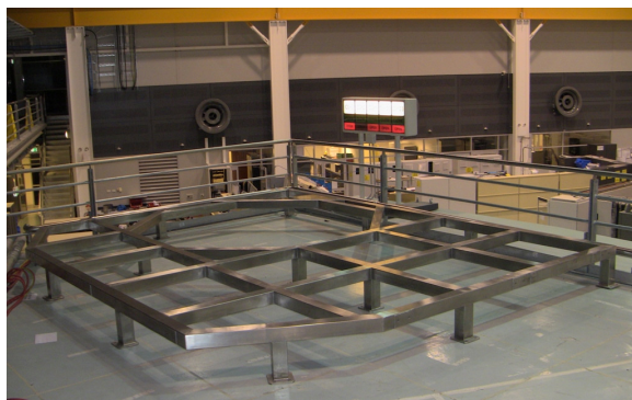
The 3 He lab support in place above the neutron cold guides.
